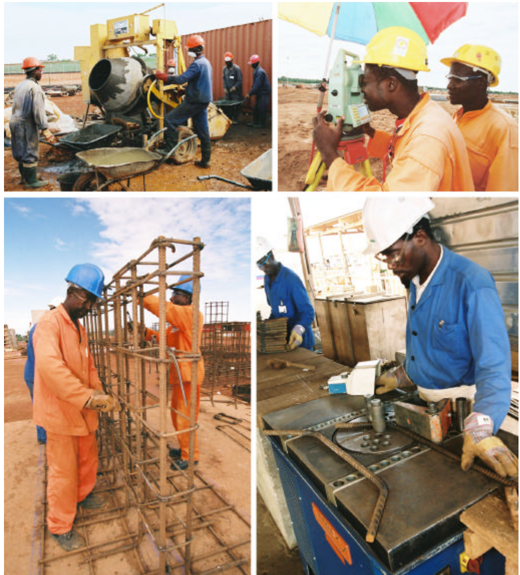
These Cameroonian workers have been hired by the facilities contractor to help build Pump Station 2, near Dompta, Cameroon.
