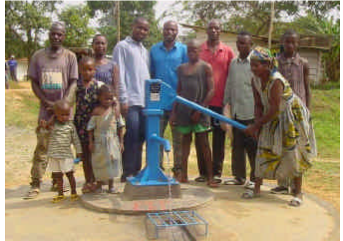
Figure 10E. A new potable water well installed in the village of Kanga, Cameroon as part of the community compensation program.
